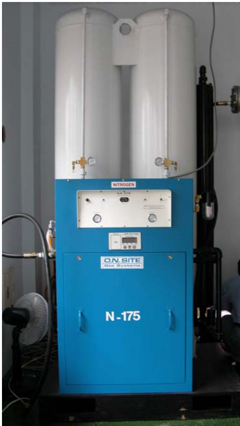
ON SITE Nitrogen Generator
